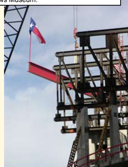
An image of the topping out of the Margot and Bill Winspear Opera House.
